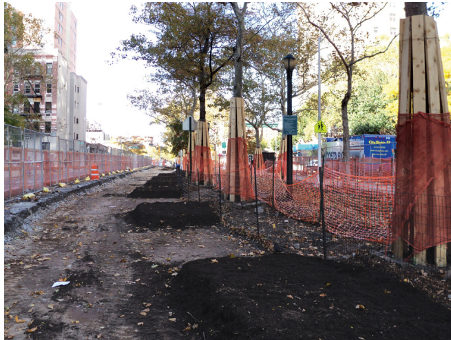
Tree protection measures during reconstruction of the Allen Street Malls, Manhattan (Credit: Parks)
